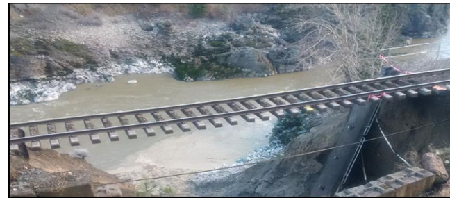
Damage from extreme precipitation in the Fraser Canyon (Nov. 2017)
