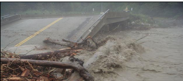
Bridge failure isolated Stewart, BC (Sept. 2011). Cost= $7M response, $11M repair
